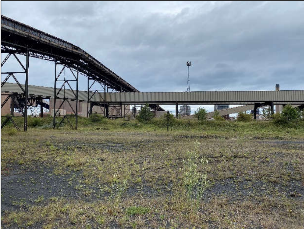
Photograph 3 - Area 10 Conveyor Belts
